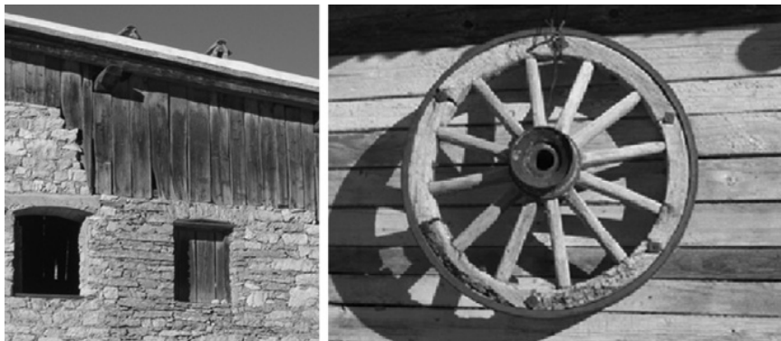
Figure 6 Examples of wood degradation.
